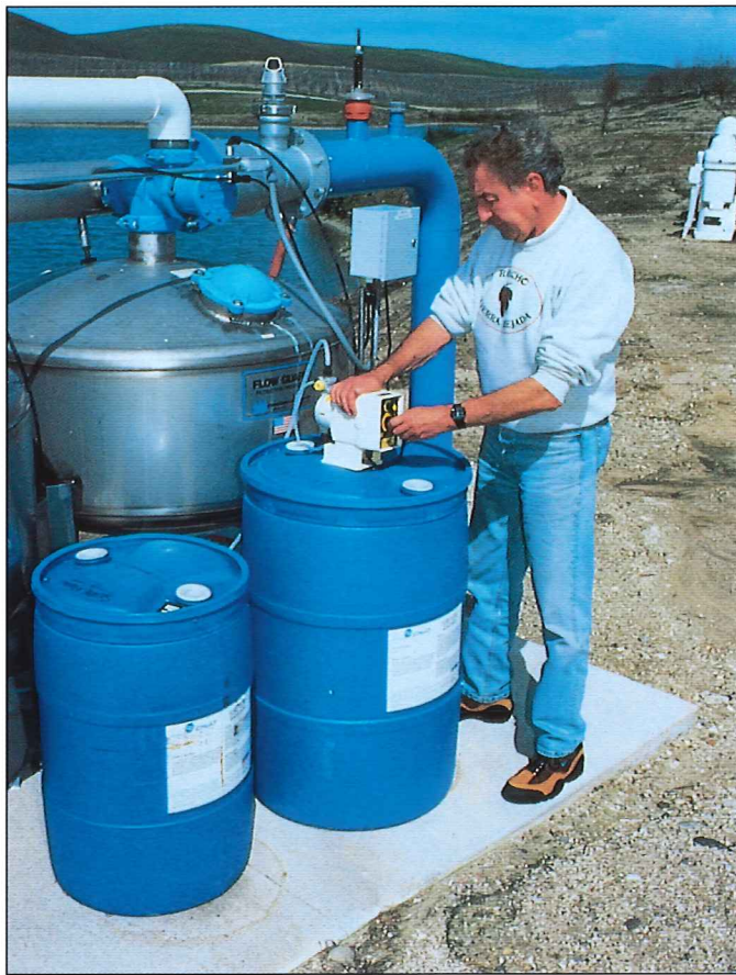
Herman Schwartz, owner of Continental Vineyards, adjusts an injection feed pump that regulates the ratio of water treatment formulation to gallons of water per minute. Photos courtesy: CH 2 O International.
